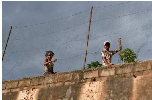
Figure- 14 grillage abimé
